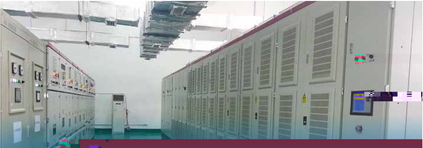
Project name: Guangxi large-scale paper-making enterprise synchronous motor special converter drive pulp mill project Application Scenario: Pulp Mill for Paper Making Industry Project highlights: 20000kVA motor, using Zhiguang high-voltage inverter one-two start-up solution, can achieve an annual output of 1.5 million tons of raw pulp and 2.5 million tons of paper.
